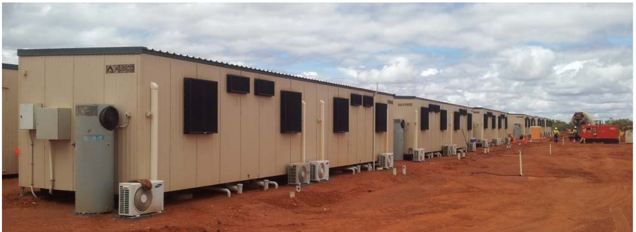
Installation of the Construction Camp is on track for completion in March.
